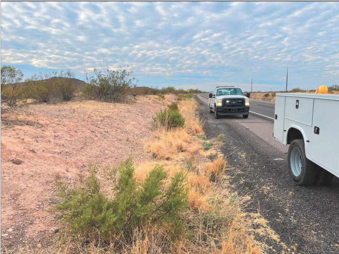
Figure 2 - Cut slope location SR 79 MP 140.7 to 140.8 with maximum height of 4 feet above roadway grade
