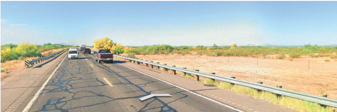
Figure 3 - Typical embankment fill location - MP 144.0 to MP 144.1 with maximum depth of 4 feet below existing roadway grade
